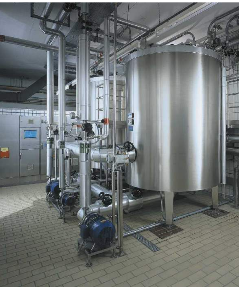
WFI storage and distribution system
